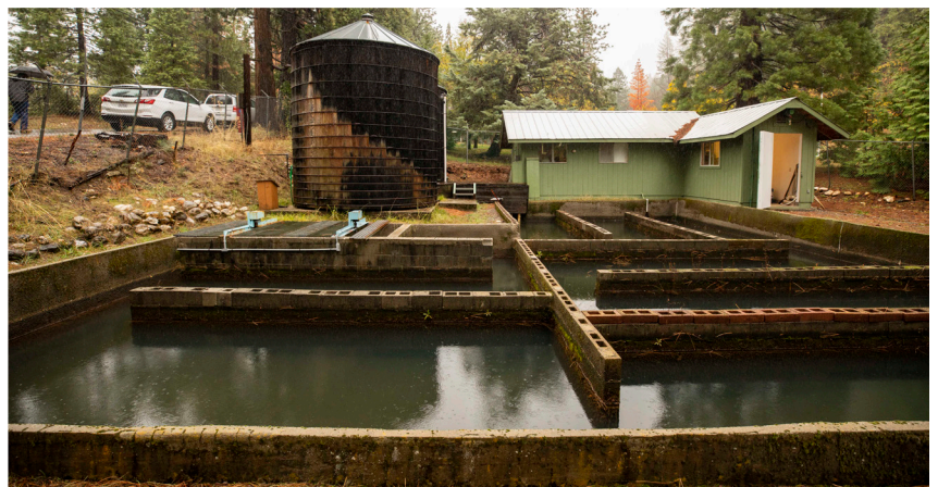
Dutch Flat Mutual Water Company's water treatment plant and basins
