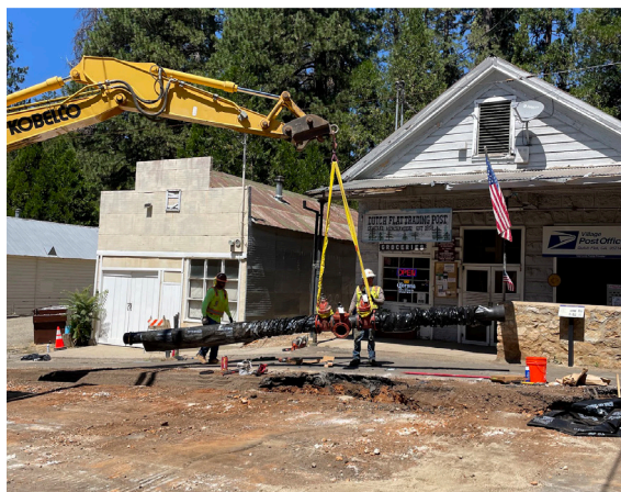
Installation of treated water pipe and a fire hydrant along Main Street
