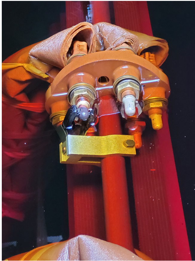
Close-up of the transformer shows carbon deposits and evidence of arcing (as seen by the dark color on the left).
