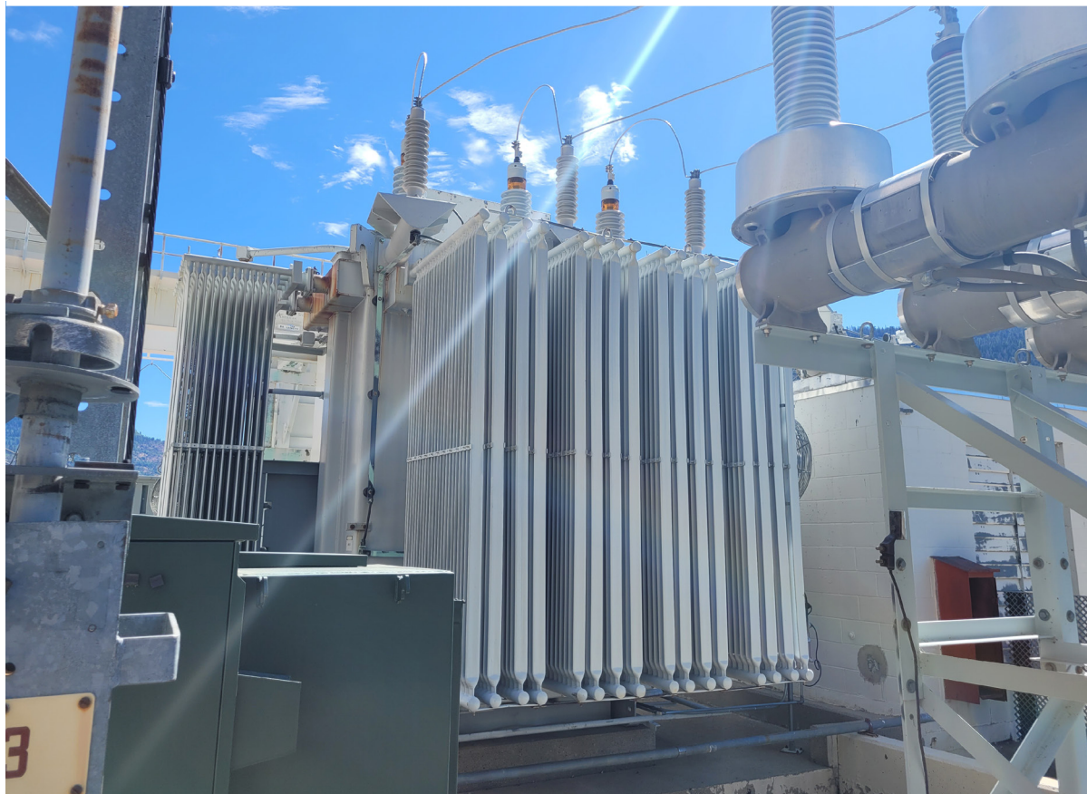
Exterior of the French Meadows Powerhouse Step Up Transformer.
