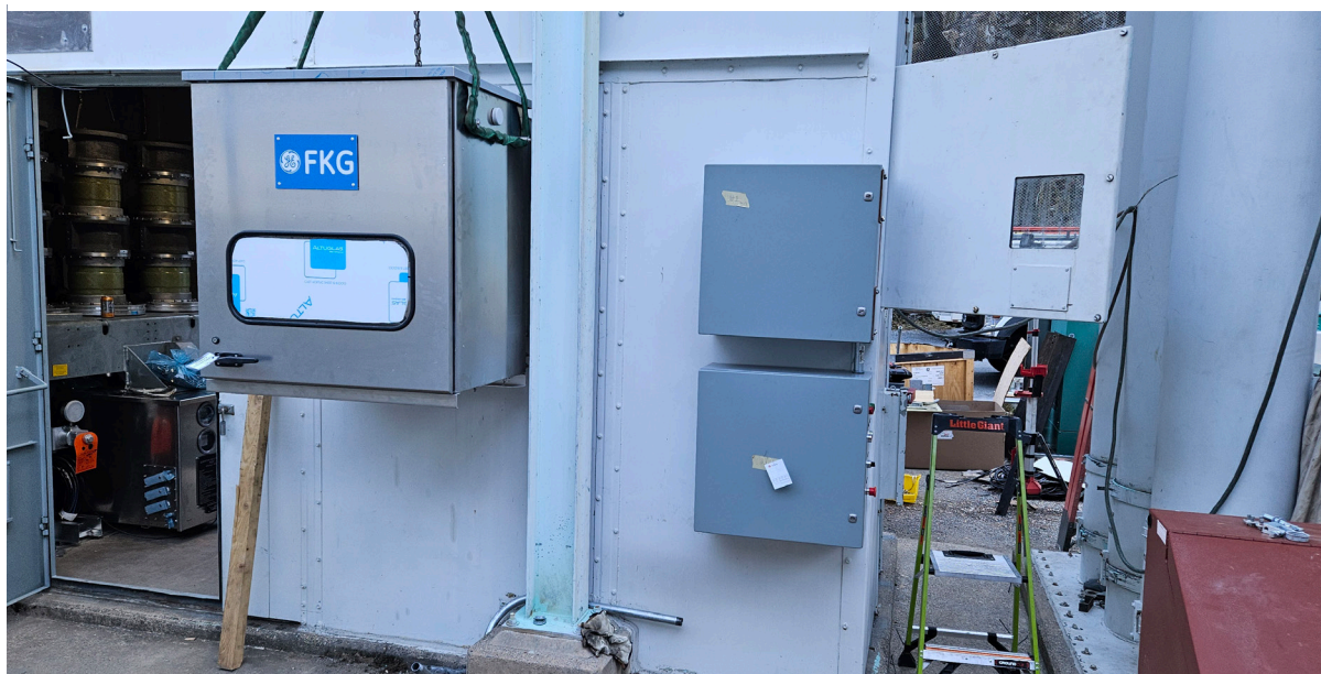
Installation of Breaker No.1 control panel in progress; Breaker No. 2 is visible inside the breaker enclosure.
