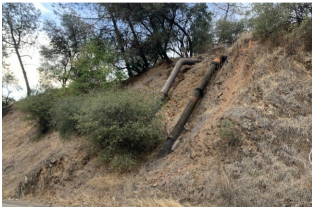
The existing raw water pipelines at Ophir Road in the Duncan Hill community.
